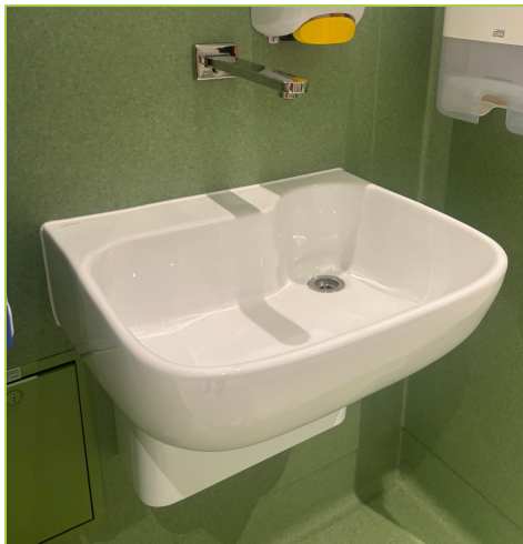
STERISAN® Basin installed at Paula Fox Melanoma & Cancer Centre
