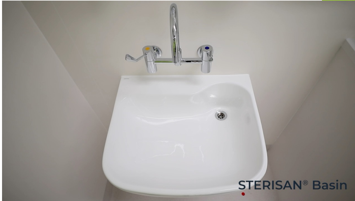
Basin & Tapware installed at Maitland Hospital
